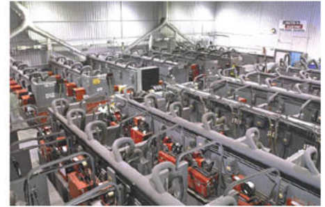
Figure 1. These welding hoods are used to exhaust a large area.
