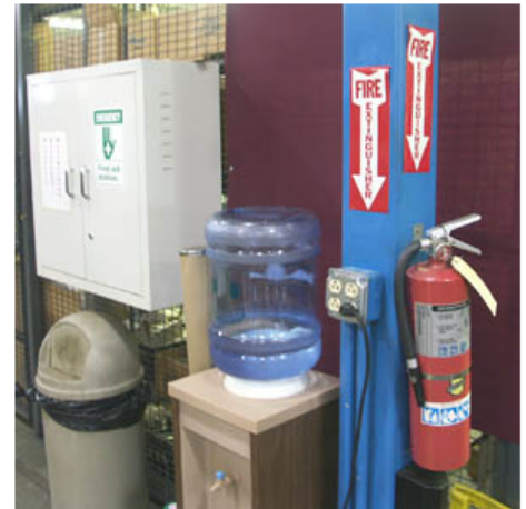
Figure 1. Fire extinguishers should be conveniently located.
