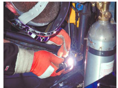
Figure 2. This welder is using arc welding to join parts without a filler metal.
