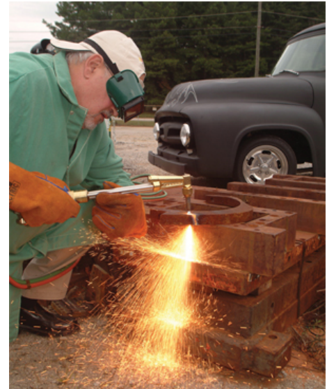
Figure 2. Working in an outdoor environment can cut down on the dangers of oxyfuel welding.
