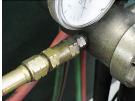
Figure 2. Hose connections should be wiped down to ensure that no gases are leaking from them.
