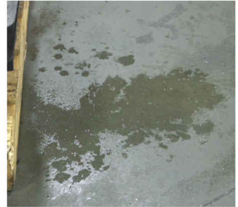
Figure 1. Wearing PPE protects against unexpected hazards like this spill..
