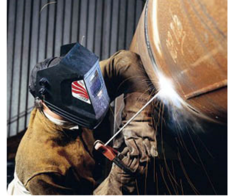
Figure 1. This welder is trained to properly use a welding helmet and other important PPE for this specific industry.
