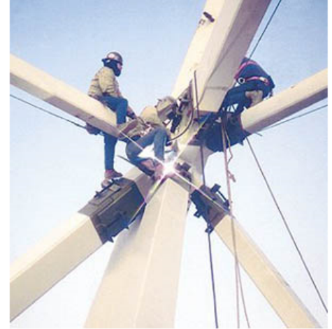
Figure 1. Failure to wear the proper PPE can result in accidents, injury, illness, or death.
