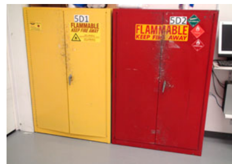
Figure 2. Section 7 of the SDS details safe storage methods for hazardous chemicals.
