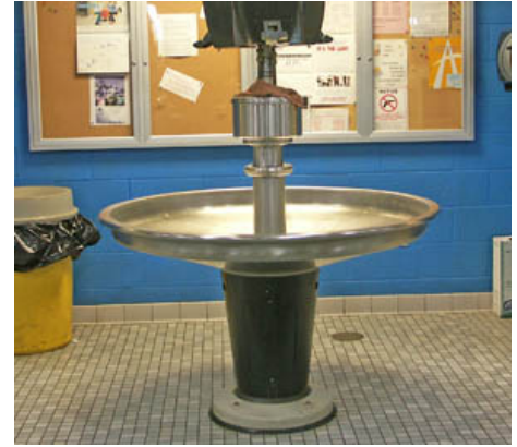
Figure 1. Employees must know the location and proper use of the hand and eye wash stations.
