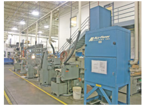
Figure 2. Work areas must be organized, and walkways must be free from obstruction.
