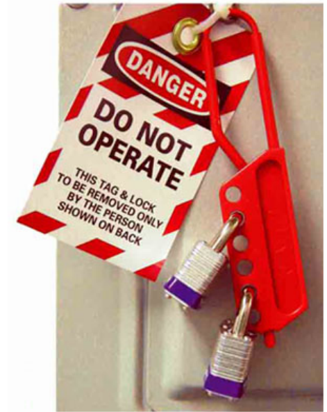
Figure 1. Electrical and mechanical devices should be put under lockout/tagout to prevent accidental startup of equipment. (Courtesy of NMC.)
