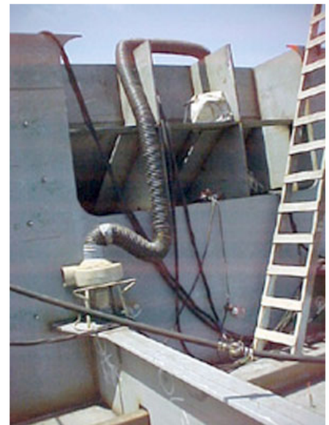
Figure 1. Exhaust fans with hoses are often used to purge and ventilate hazardous atmospheres.
