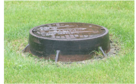
Figure 1. Written programs must include procedures for appropriate testing of atmospheric hazards, such as the gases that might be present in this manhole.
