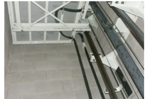
Figure 2. An elevator shaft is usually considered a confined space because it is a pit with only one means of entry.
