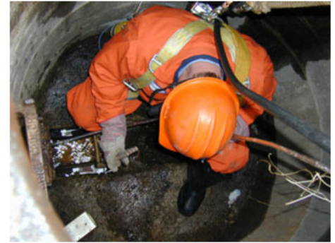
Figure 1. The authorized entrant is the person trained to enter the confined space.
