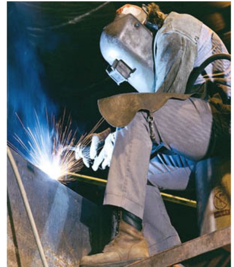
Figure 2. Welding inside a confined space can expose workers to fumes, heat, explosions, and other hazards.
