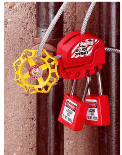
Figure 2. Isolating valves to keep substances from entering the confined space is among the preparations necessary for entry.
